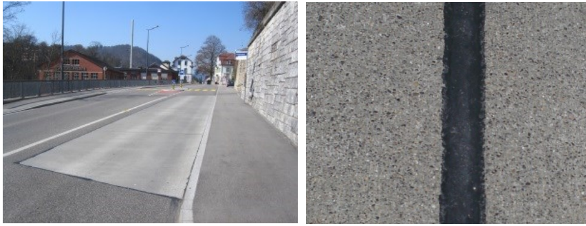
Figure 20: Concrete elements at a bus stop (left) and close-up of a joint between two noise-optimised concrete elements (right) (Source: [25], modified by Grolimund + Partner AG)
